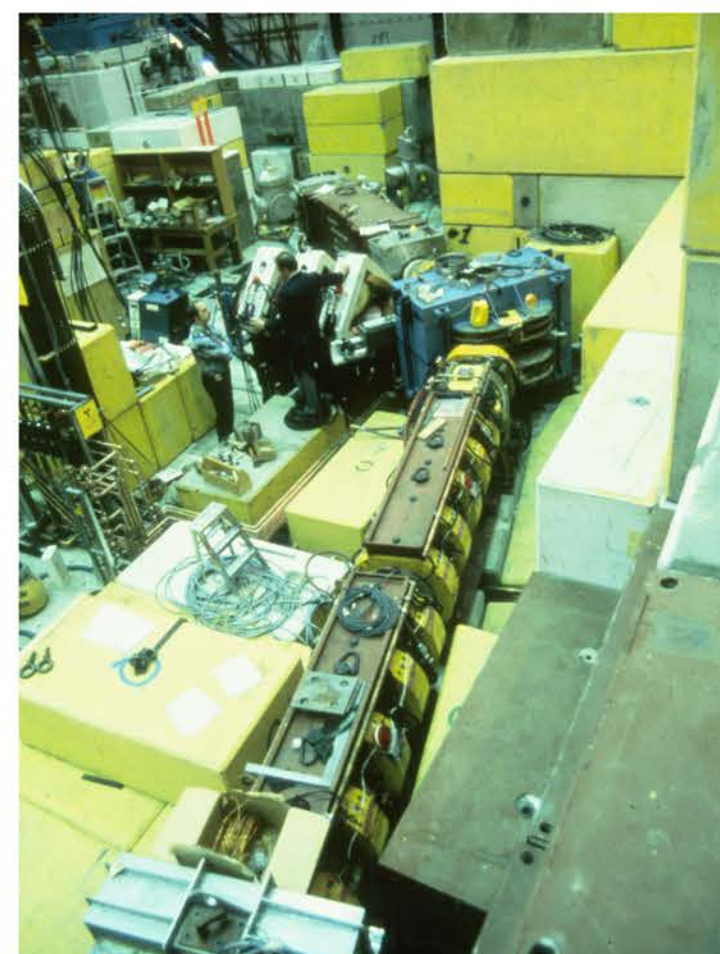
The M20 beam line (circa 1986) in the Meson Hall provides muons for \mu SR studies in condensed matter physics and Mu chemistry. Recently upgraded (2013). Image source: TRIUMF.
