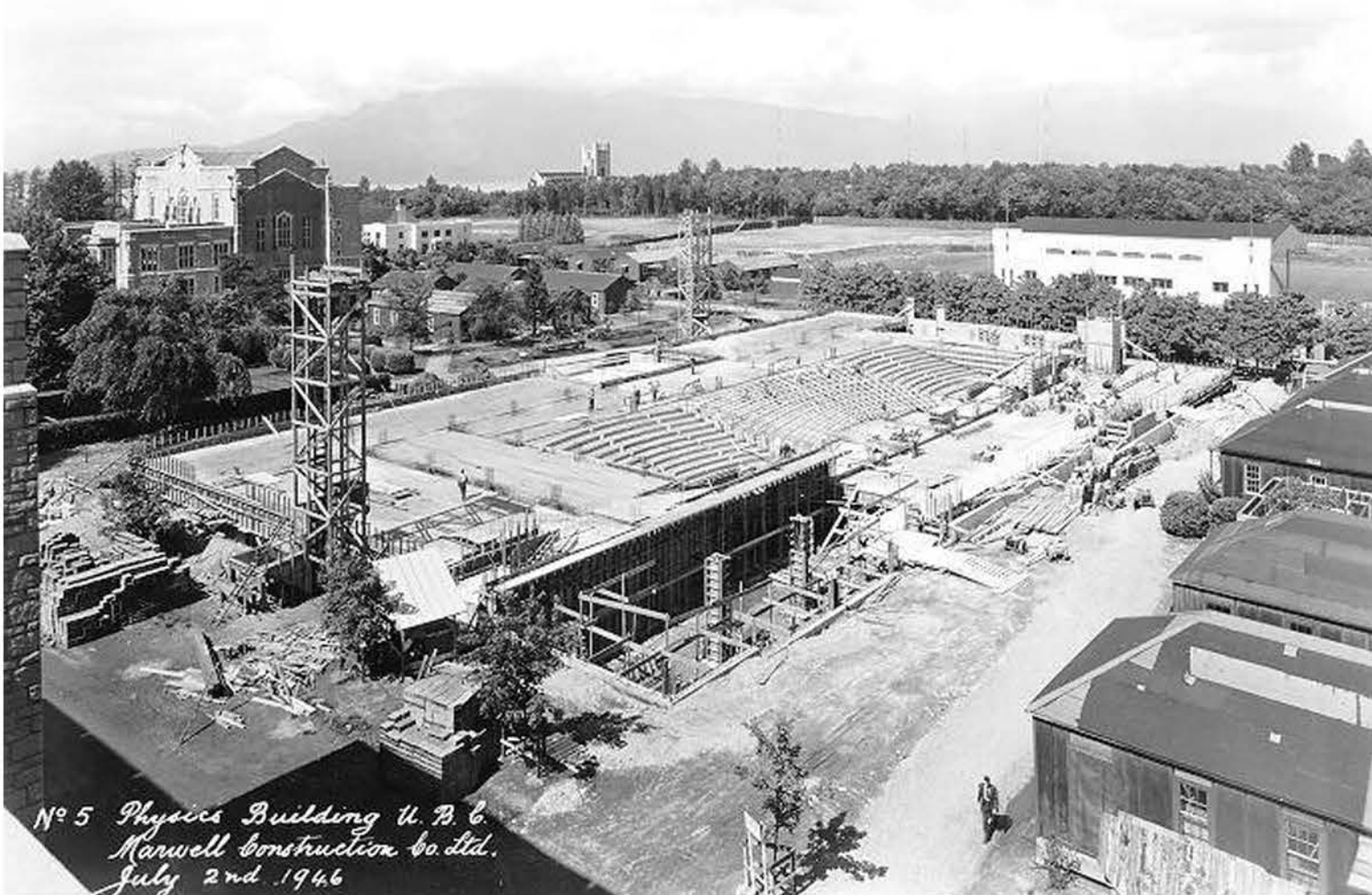
Construction photograph of 1946 showing the location of lecture theatres. L-R: Hennings 202, 200 and 201.
